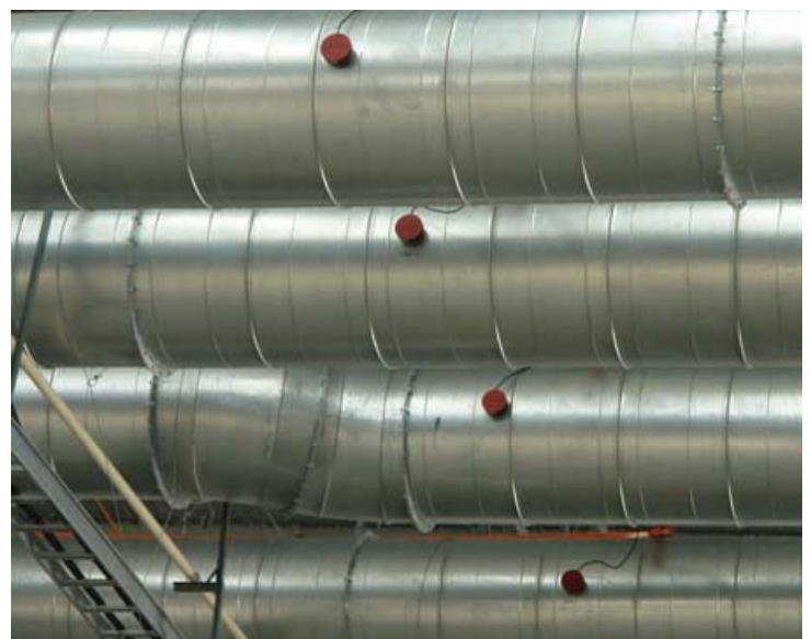
Spark Detectors Applied to an Array of Horizontal Ducting
